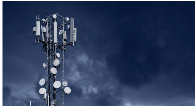
Telecom and Data
